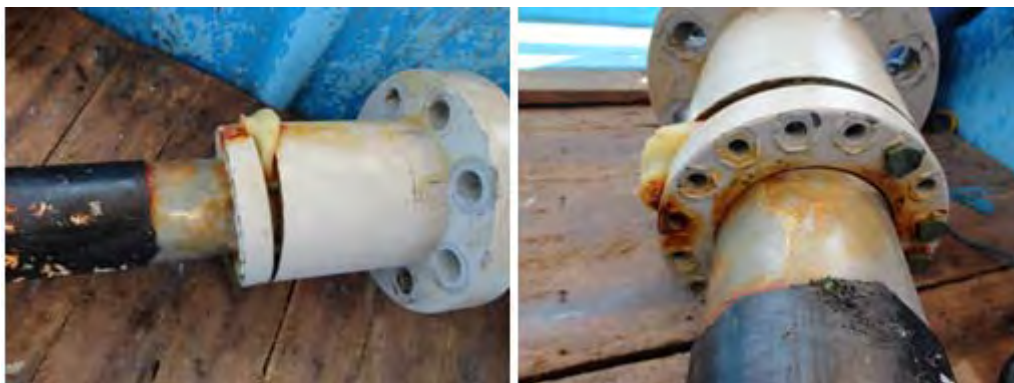
Fig. 4 Damaged smart flanged removed from the sealine
